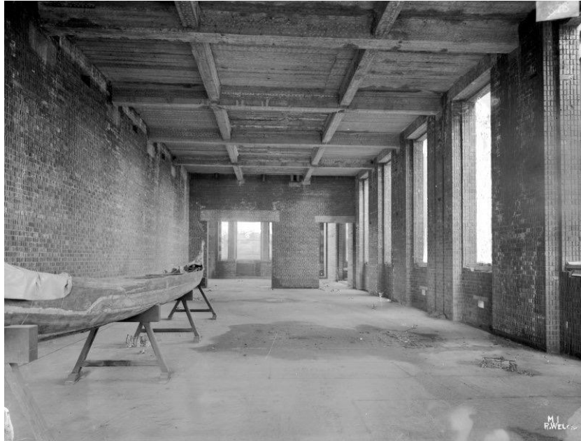
Fig. 24. 1925. Belfast Museum and Art Gallery, Stranmillis Road. The canoe is now in what, during Winifred Glover's era, was to become the Ethnography Gallery (colloquially described by her as the 'Boat Room'), while it is under construction. The end of the prow has not yet been re-attached to the canoe following the move to the new museum site. The crocodile mouth is at the prow end. Clear damage is shown by white markings, not present in the earlier photographs. This demonstrates that the damage did not, as suggested by the museum's Accession Register, occur as a result of 'storms en route' while in transit from the Solomon Islands. BELUM.Y.W.10.79.3. © National Museums NI.
