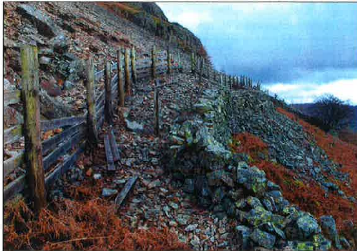
Figure 1. Wall above the Old Dungeon Ghyll Hotel in Great Langdale overtopped by downslope movement of talus.
