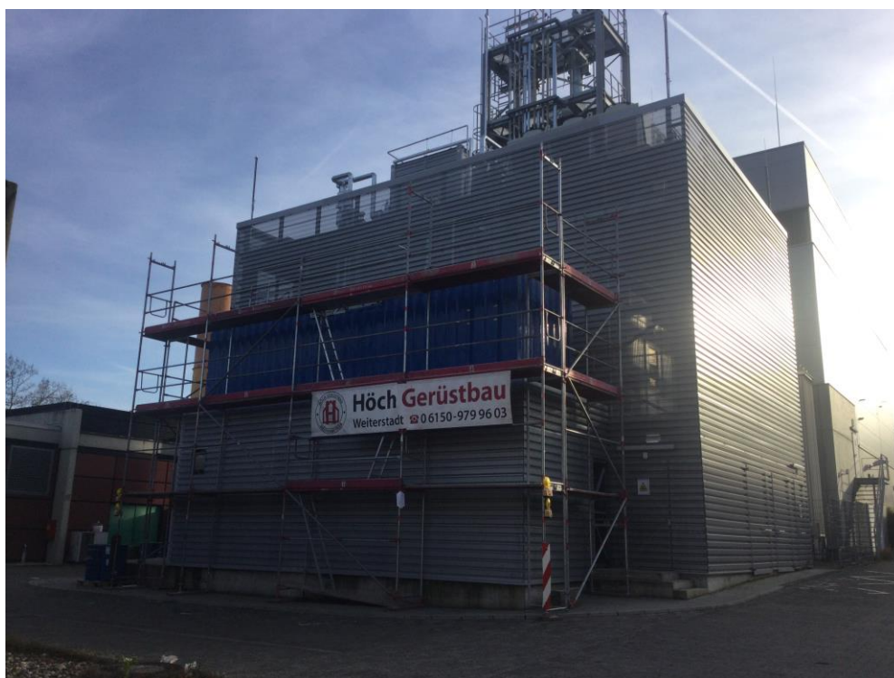
Figure 7: Image of the novel gas treatment plant (background) and the two RWE test rigs (lower container behind cladding: fuel synthesis test rig, upper container: gas treatment test rig).
